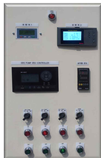
MFCQ installed on panel
